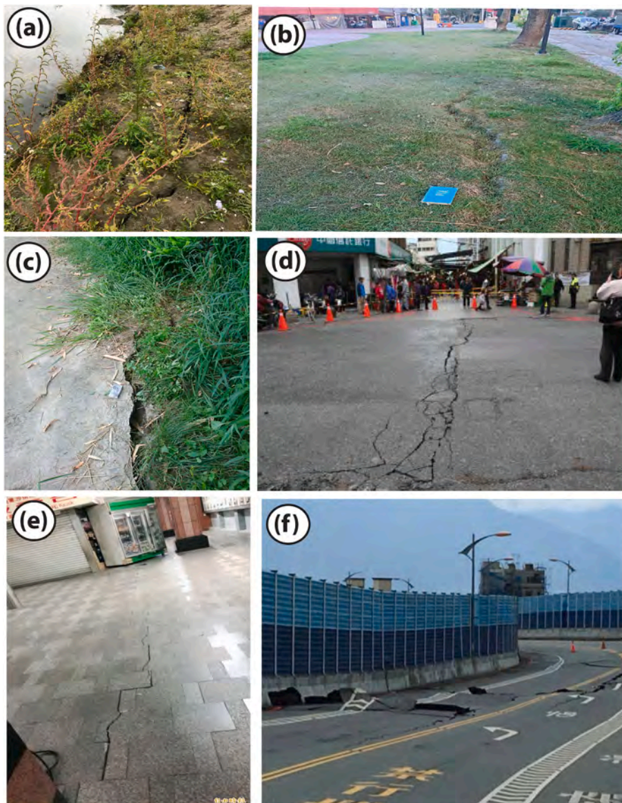
Fig. 7. Field photographs showing observed cracks during February 6, 2018 Hualien earthquake. (a) Surface cracks observed along the south bank of Meilun River. (b) 10 cm wide and several meter-long surface cracks at the night market, Hualien city. (c) Several meter long and 8 cm wide tensional cracks at north of the Mingli elementary school. (d) Crack observed on road near the Marshal Hotel. (e) Cracks on the platform of the Hualien Railway Station. (f) Observed cracks at the Chihsingtan Bridge (Photo: Huang et al., 2019; Fischer et al., 2018; https://news.ltn.com.tw/news/life/breakingnews/233484 ; https://udn.com/news/story/6656/297361 ).
