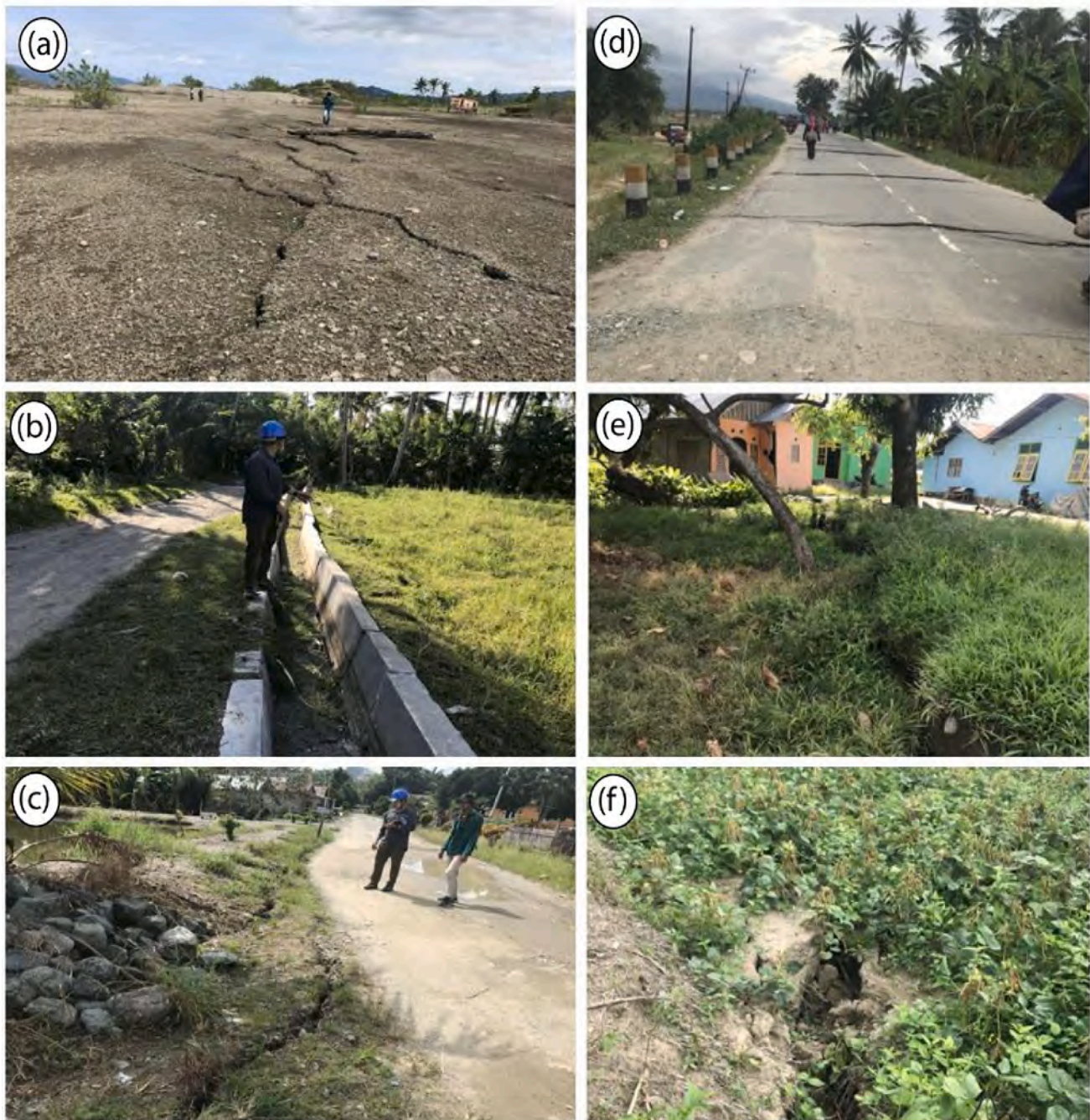
Fig. 14. Field photographs showing the ground cracks observed during the 2018 Palu earthquake around (a) Dampal; (b) and (e) Tondo; (c) Tamarenja and (d) Jono Oge, (e) Pakuli, (f) Amal.
