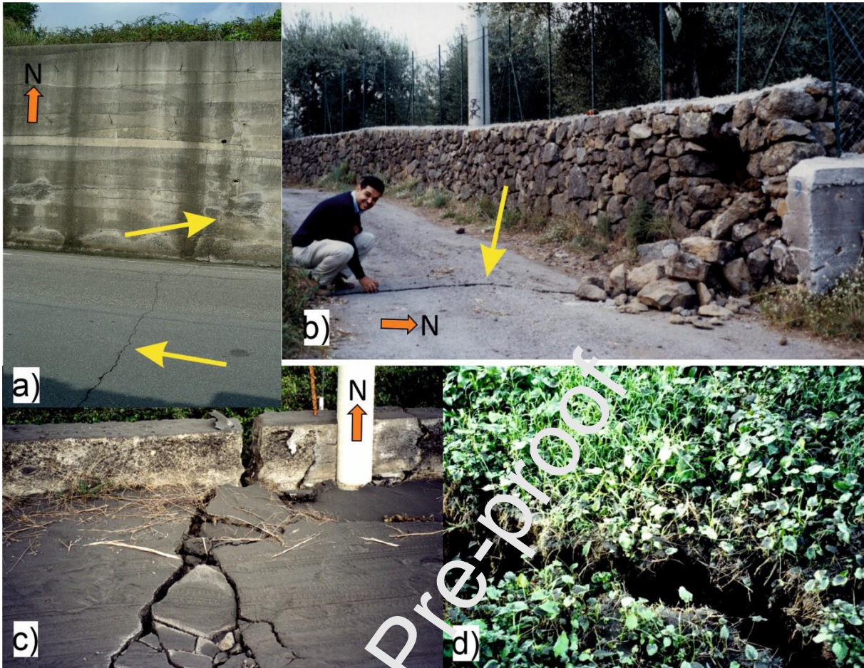
Figure 4: Field photos (taken between 29-31 October, 2002) of the surface ruptures related to the Santa Venerina and Scillichenti earthquakes, locations in figure 3. a) ground break along a road and a concrete wall in the W side of Santa Venerina; b) ground rupture on a secondary road and collapse of a dry wall; c) ground cracks affecting a road and a wall in the NW side of San Giovanni Bosco; d) large crack on the soil to the S of Scillichenti.
