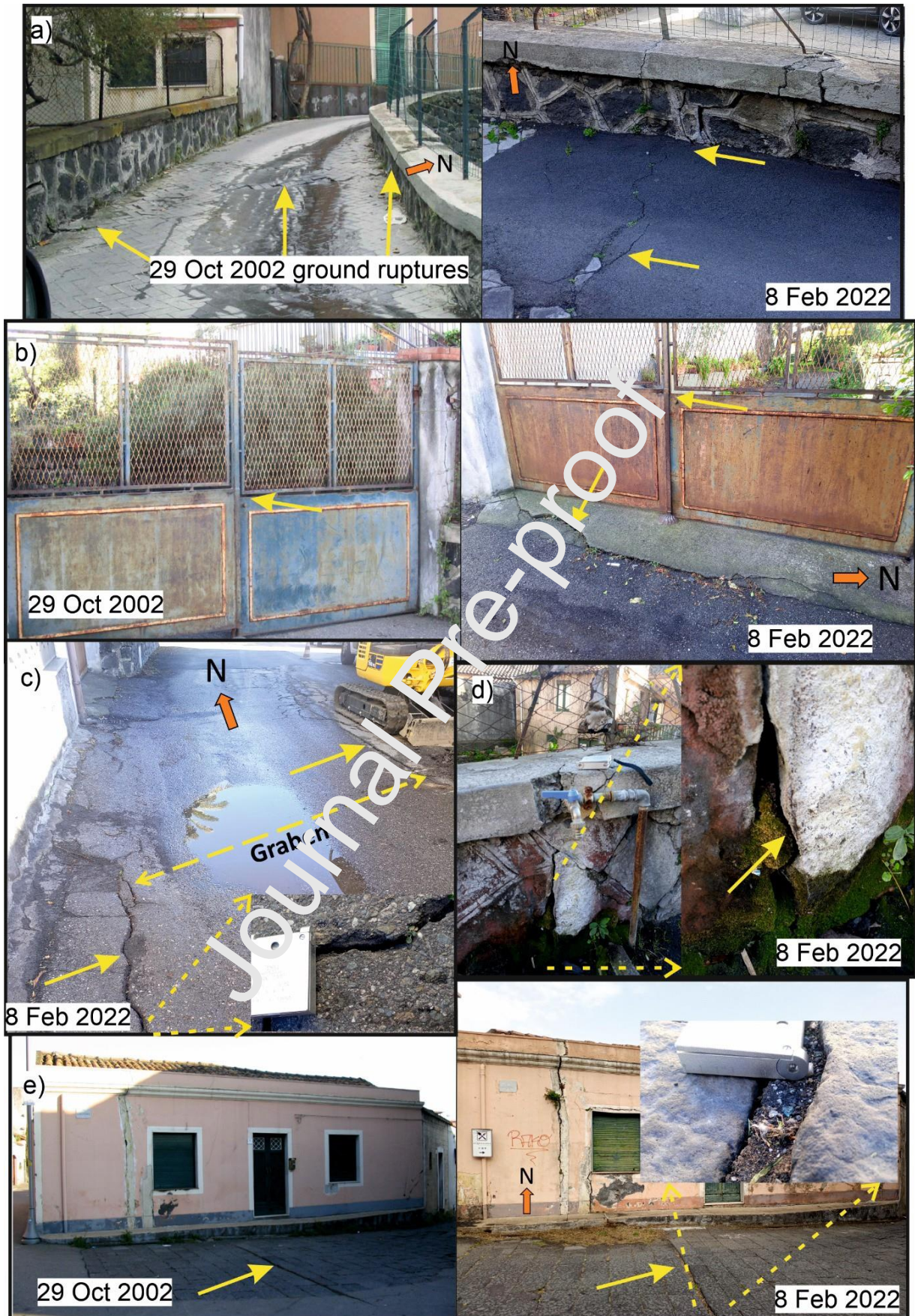
Figure 7: Field photos of the ground breaks (see blue points in Fig. 6 for location): a) fractures on pavements and walls of a secondary road; b) gate displaced by the fault creep; c) main and antithetic faults delimiting a graben; d) fracture on a wall with displaced masonry; e) building damaged and accumulated displacement between the road basaltic tiles.
