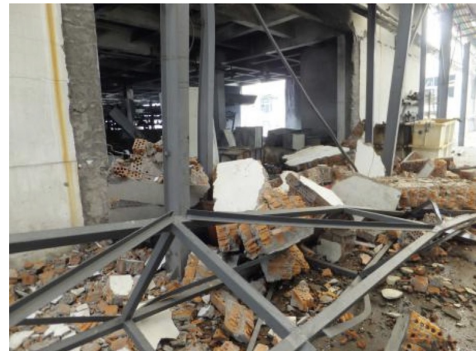
(d) A wall of the facility destroyed by the catastrophe
