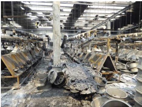
(c) Second floor after the explosion
