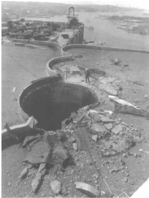
Figure 2.4: Picture of the silo roof after the wheat grain explosion (Source: Eckhoff R.,2003)
