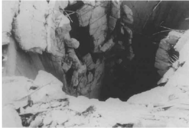
Figure 2.5: Picture of the air shaft along the damaged walls of reinforced concrete silo cells of the grain terminal (Source: Eckhoff R.,2003)
