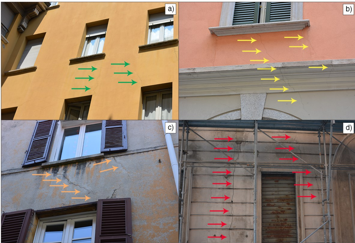
Figure 3.5. Modified from Nappo et al. (2021a). Building damage severity classification adapted from Burland et al. (1977): a) negligible ( w < 0.1 mm - D1); b) very slight ( w < 1 mm - D2); c) slight ( w < 5 mm - D3); d) moderate ( w > 5 mm - D4). Field investigations were performed in June 2019.
