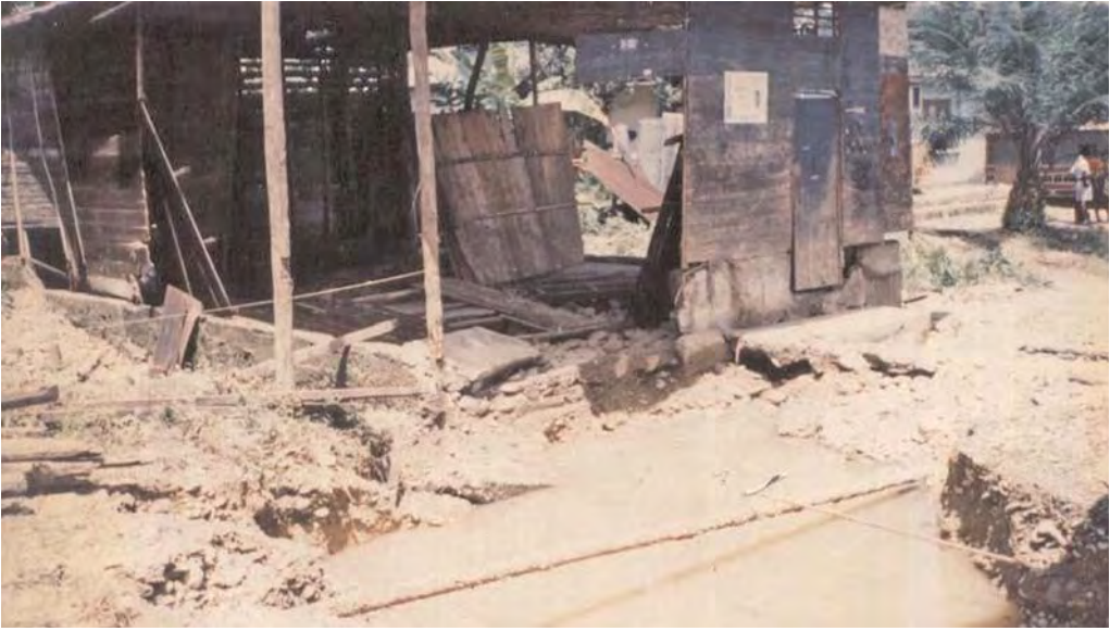
Fig. 10. Liquefaction with water upsurge in la Grande, Rio Sucio (photo: S. Mosquera-Machado).
